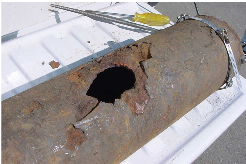
FIGURE 1.3.2 A failed cast iron pipe. Courtesy of Mark Lewis, East Bay Municipal Utility District.
