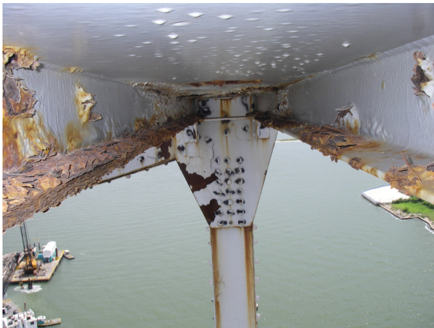
FIGURE 1.3.1 The underside of a steel bridge member exhibiting significant corrosion. Courtesy of the Texas Department of Transportation, © 2007. All rights reserved.
